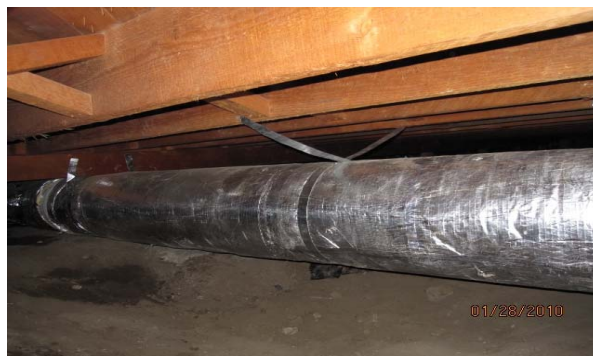
New ductwork in crawl spac
