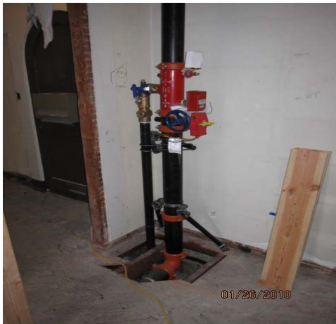
New Sprinkler System Fire Riser
